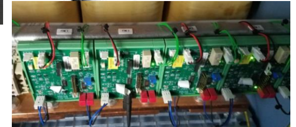
Flow switches located internally in MPS
