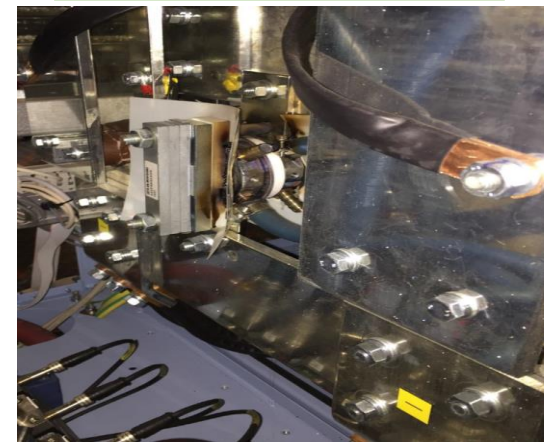
Disconnected hoses on SCR at Torus MPS
