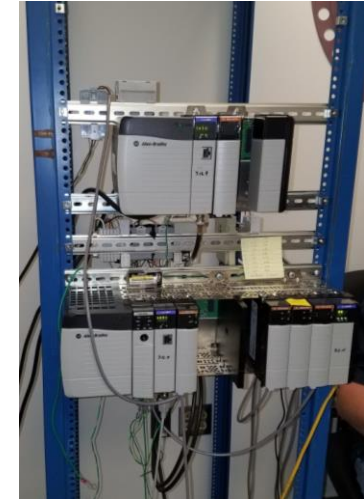
Stand-alone PLC setup used for Ethernet/Controlnet compatibility test
