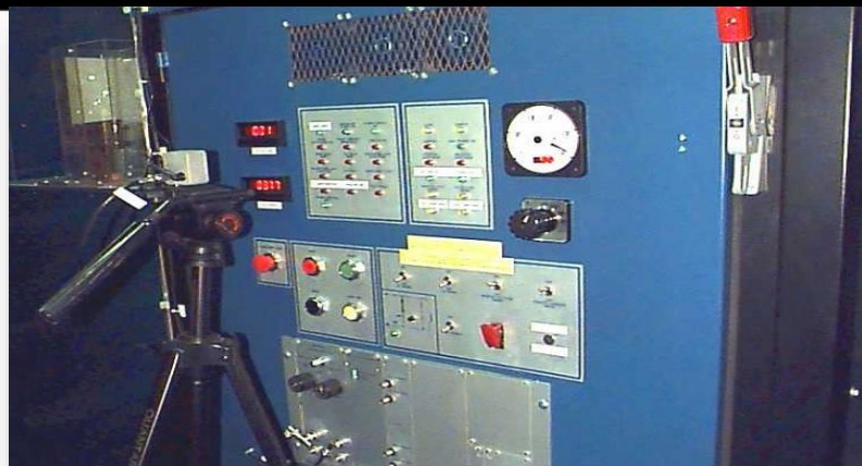
10 V, 2000 A DC Dynapower dipole magnet power supply
