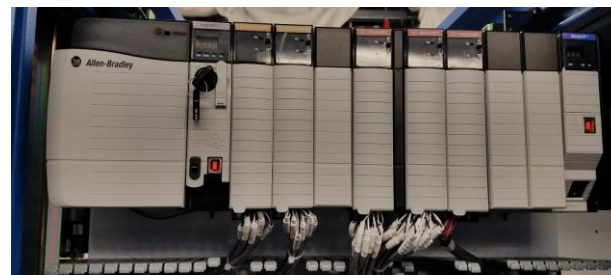
Local solenoid PLC control systems
