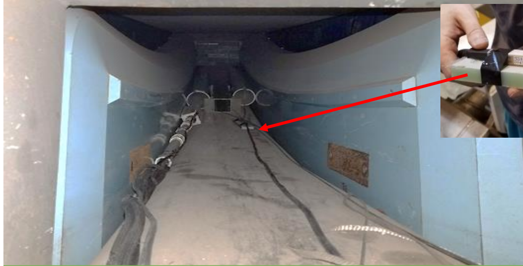
Hall probe installed inside central area of the HMS dipole
